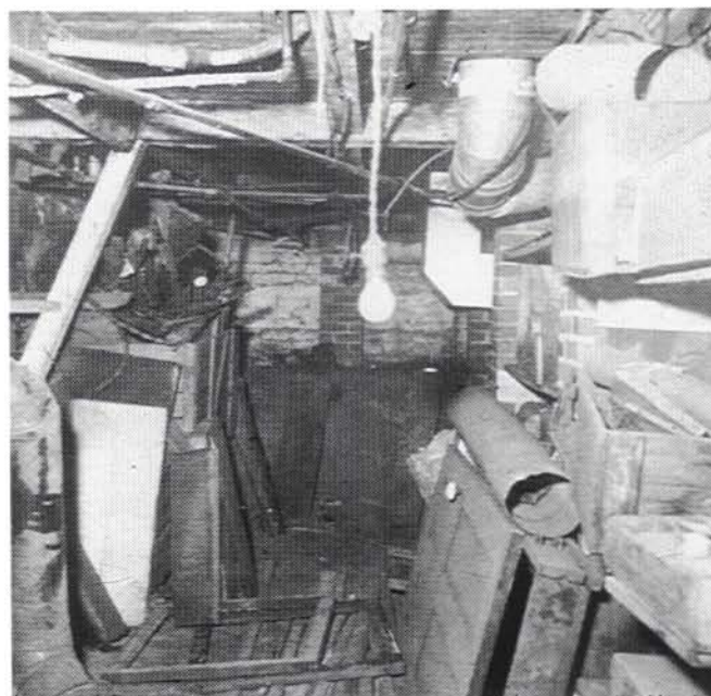
Figure F. Outdated fixtures and systems are frequently abandoned in place when more modern units are installed. Examining and documenting their existence can provide a technological reference to the history and use of many rooms or structures. photo: NPS Preservation Assistance Division Files.
