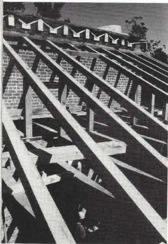
8 Roof framing showing white oak joists, posts, rafters. Note "rooflets" beneath flat central terras roof, at top of photo. In a rare divergence from the original design, the restoration team covered the rooflets with a rubber membrane to guard against leaks.
